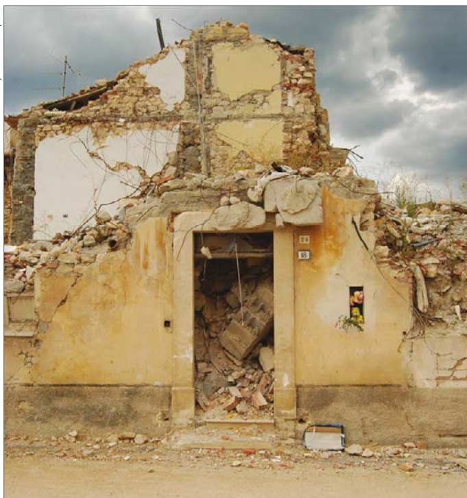
Devastated Building damage in the village of Onna, days after the L'Aquila earthquake struck Italy in April 2009.
