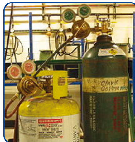
Figure 6-6. Compressed hydrogen storage
